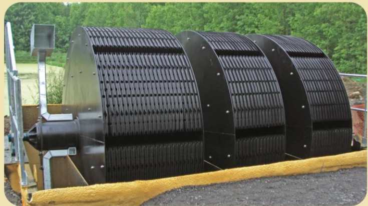
Rotating Biological Contactor (RBC) pengolahan biologis attached growth
